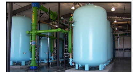
McCook Water Treatment Equipment
